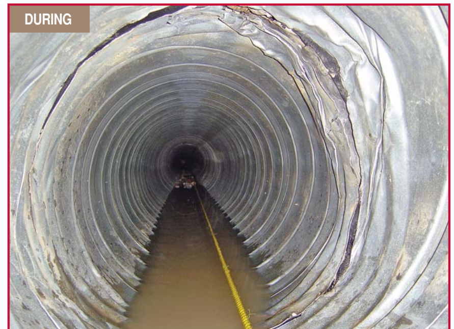
The pipe is shown after after the hydraulic cylinder pushed the corrugated metal back into place.
