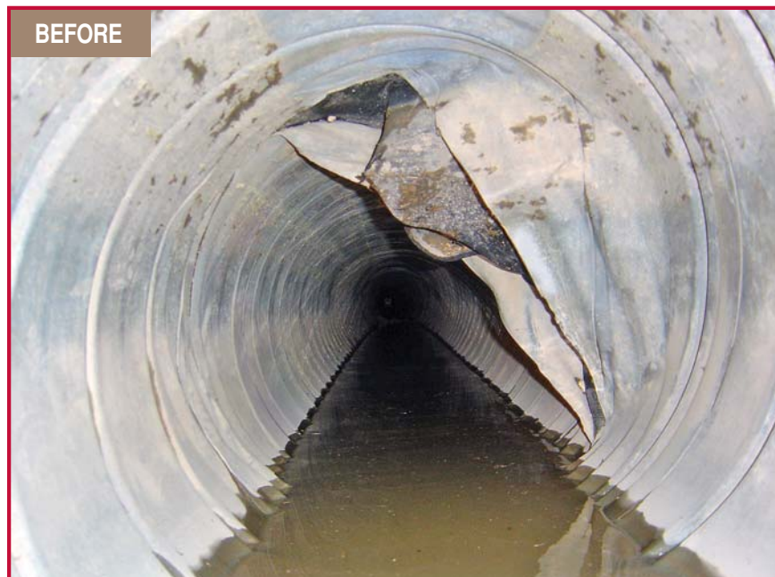
The pipe was damaged from the 11 o'clock to 4 o'clock positions, affecting one-third of the diameter. Both pipe ends splay inward, exposing the black rubber gasket. Twelve inches of water stood in the invert.
